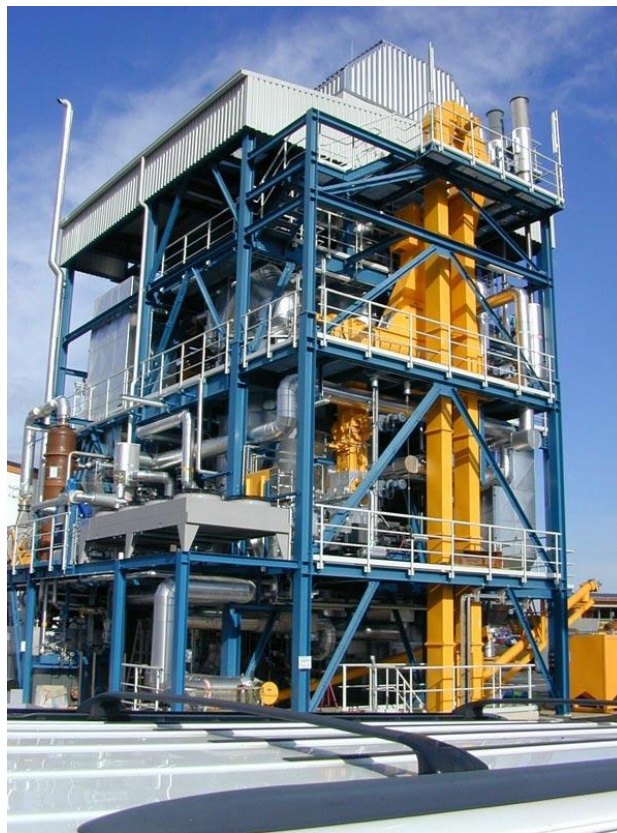
Figure 11. The Güssing Biomass Power Plant [5]
