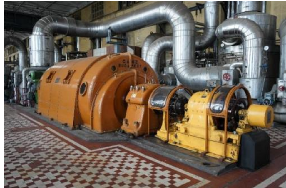
Back-pressure steam turbine generator
