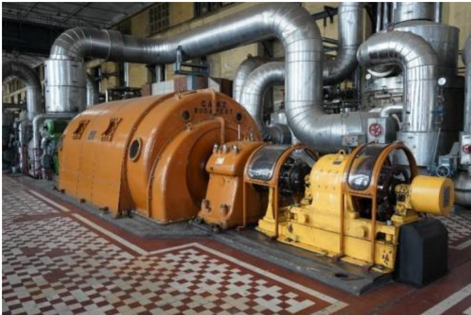
Figure 15. Back pressure steam turbine-generator (27 MW e ) [12]
