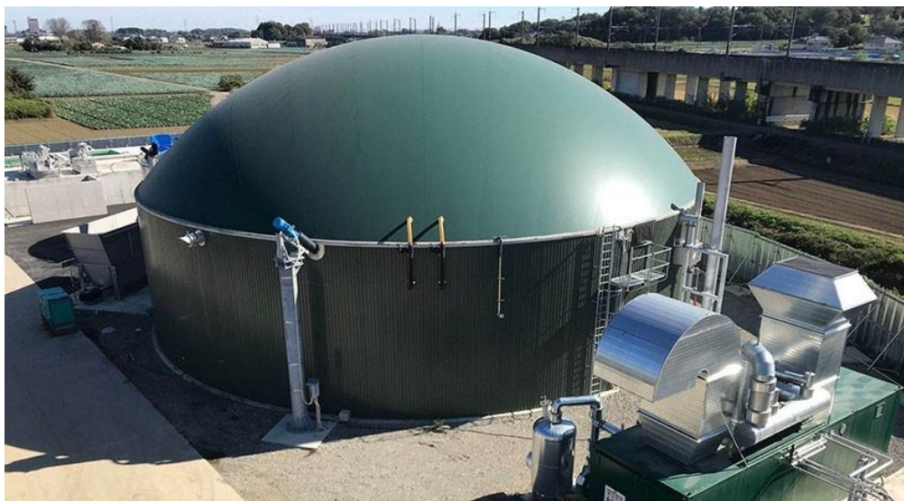
Figure 3. Biogas fermenter and gas engine [3]
