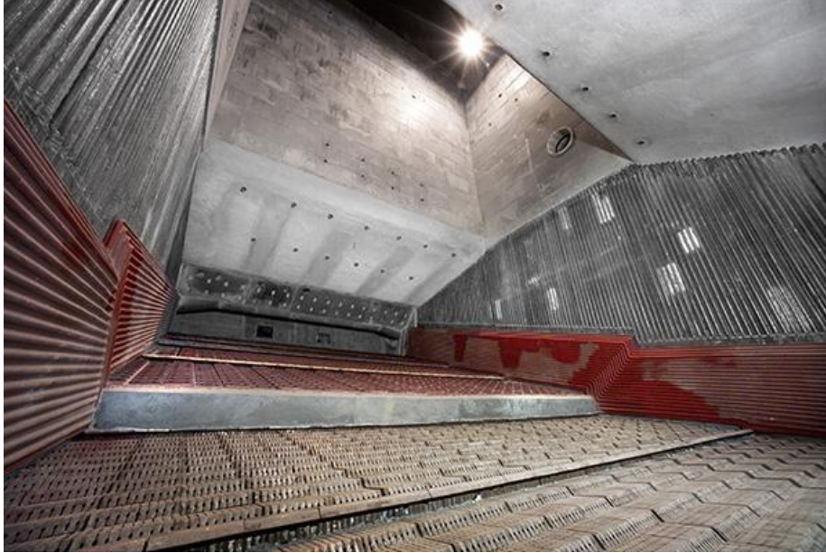
Figure 22. Grate at a WTE plant [20]
