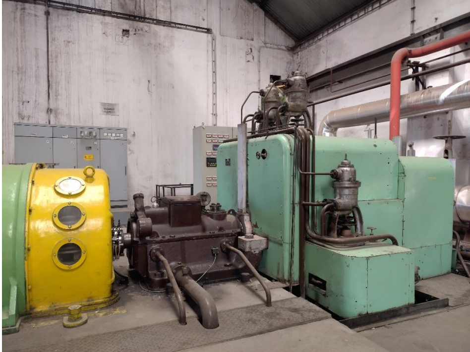
Figure 14. Back pressure steam turbine (2 MW e )
