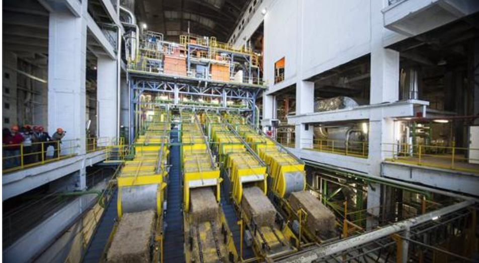
Figure 4. Straw line at biomass CHP plant [4]
