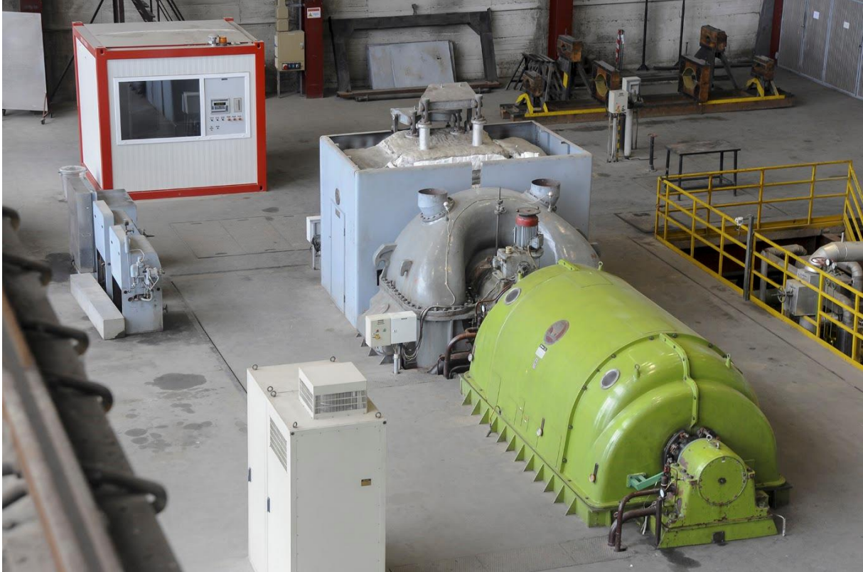
Figure 23. Extracted-condensing steam turbine at waste to Energy plant in Budapest [19]
