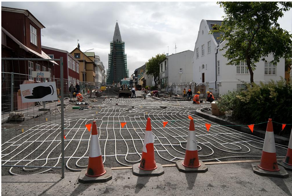
Figure 12. After circulating through the building, the excess, low-quality geothermal heat is used for road de-icing (underfloor)
