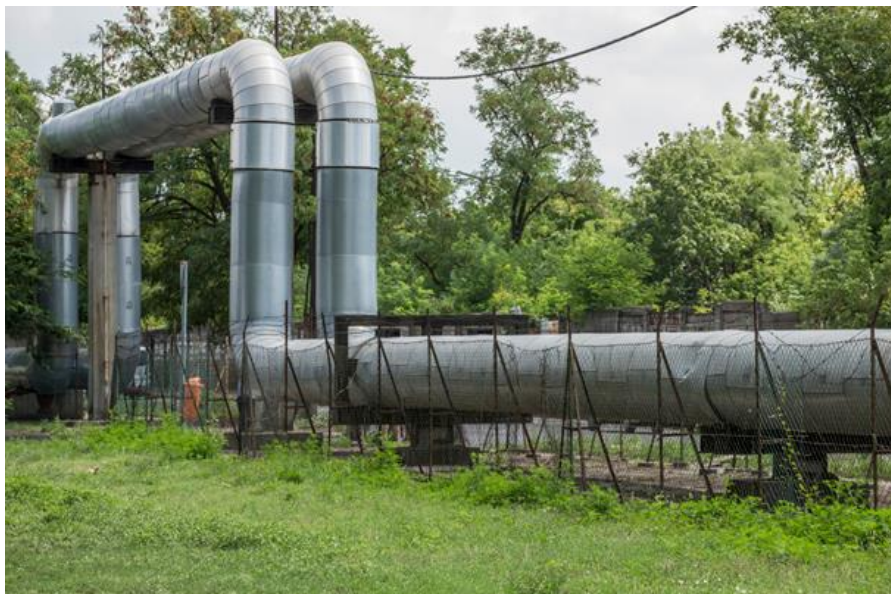
Figure 6. Overground DH pipelines (mokshahu)
