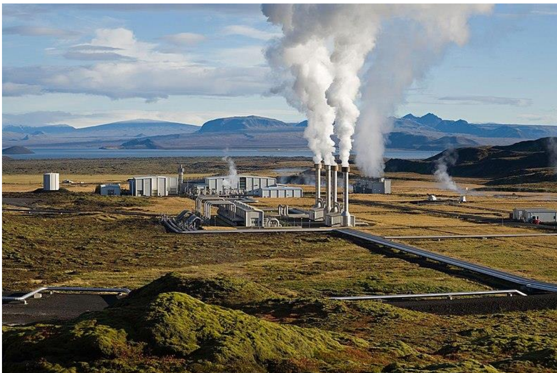
Figure 11. Iceland geothermal power plant and district heating systems (nesjavellir)
