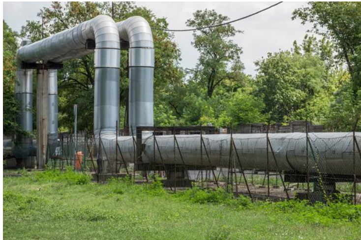
Figure 2. Overground DH pipelines [2]
